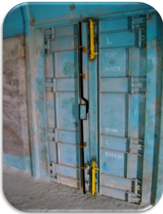
Inner view of additional door locking arrangement
