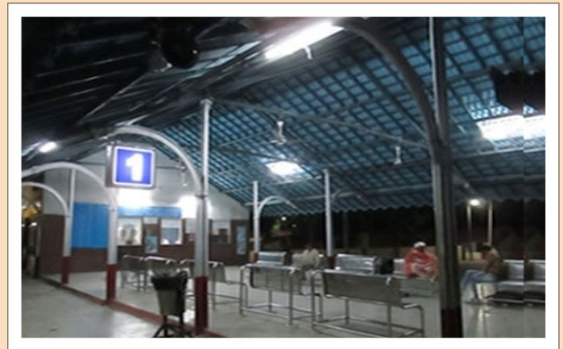
LED Lights installed at Makarpura Station
