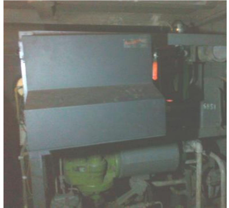
Brake Interface unit in Machine room
