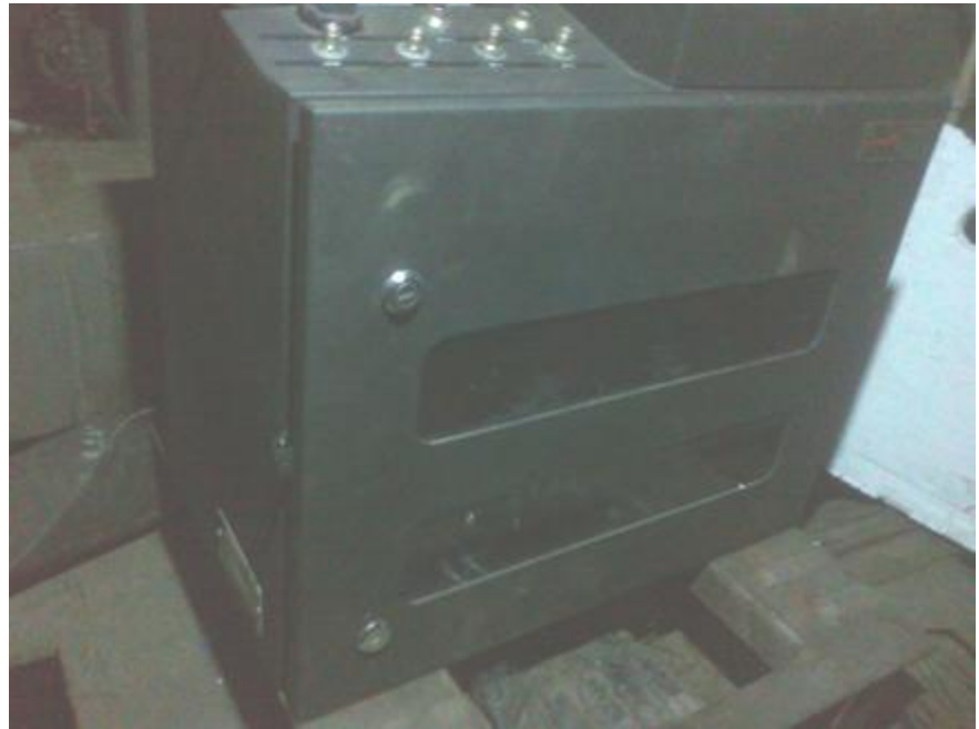
CCU In the Machine room
