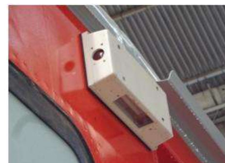
Figure 1.30 Passenger Alarm Coach Indication Light
