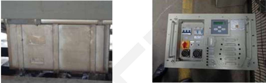
Figure 1.11 Regulated Battery Charger
