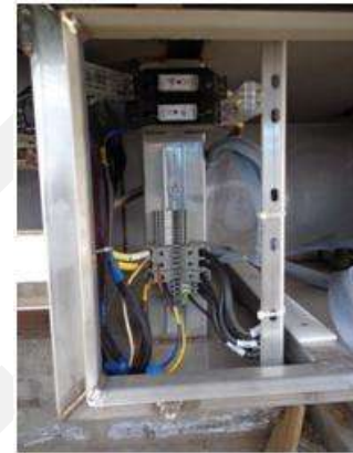
Figure 1.8 Battery Charging connection
