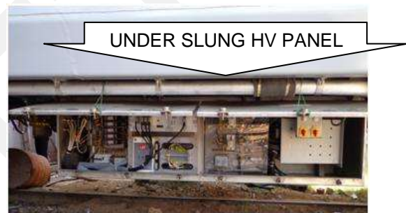
Figure 1.4 High Voltage Cubicle
