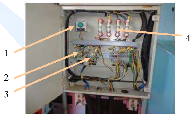
Figure 1.22 On Board Rotary Switch Panel
