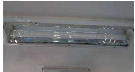
Figure 1.24 Fluorescent Light Fitting
