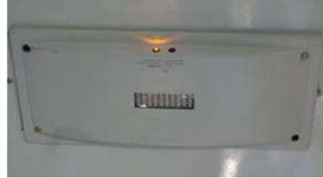
Figure 1.26 Emergency Lighting Unit
