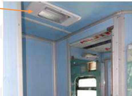
Figure 1.27 Gangway/ doorway Light
