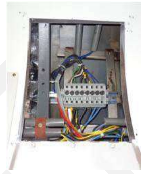
Figure 1.35 Fuse Distribution Boards
