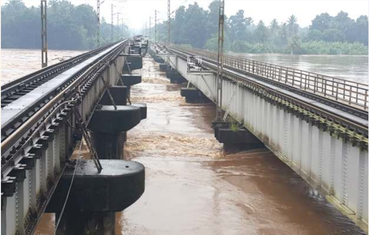
Rising Water Level under Railway Bridge
