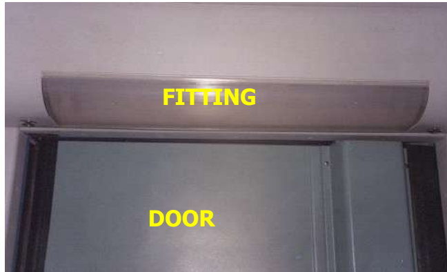
Figure 6.25 Doorway Light Fitting
