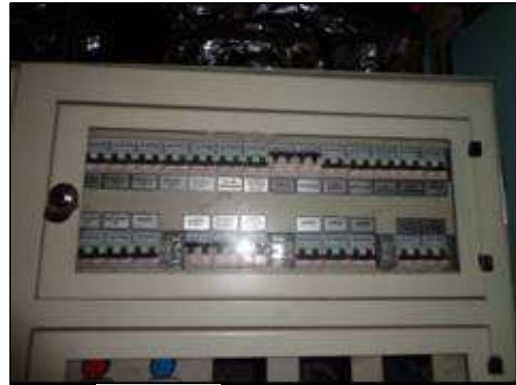
Lavatory panel light control
