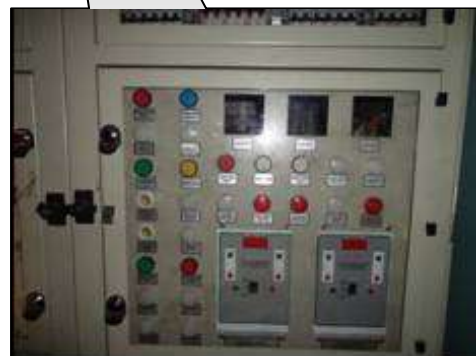
Control unit for water pump
