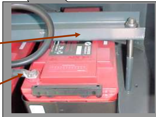
Battery Module Details
