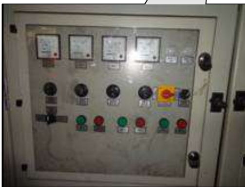
Control unit for main feeder supply and network
