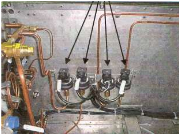
Figure 6.14 Pressure Transducers in RMPU
