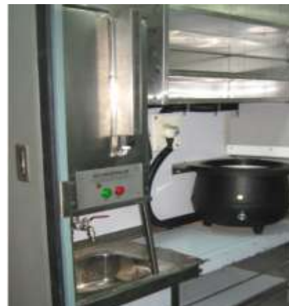
Vertical Water Boiler in Existing Design Coaches
