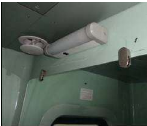
Figure Toilet Light Fitting
