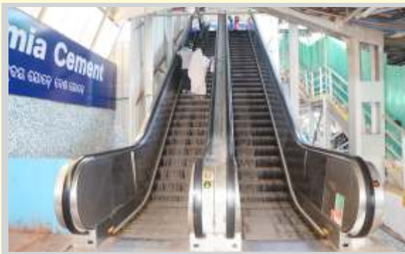
Escalator at Bhubaneswar Station
