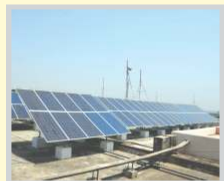
Solar Power Plant at Rail Sadan Roof Top
